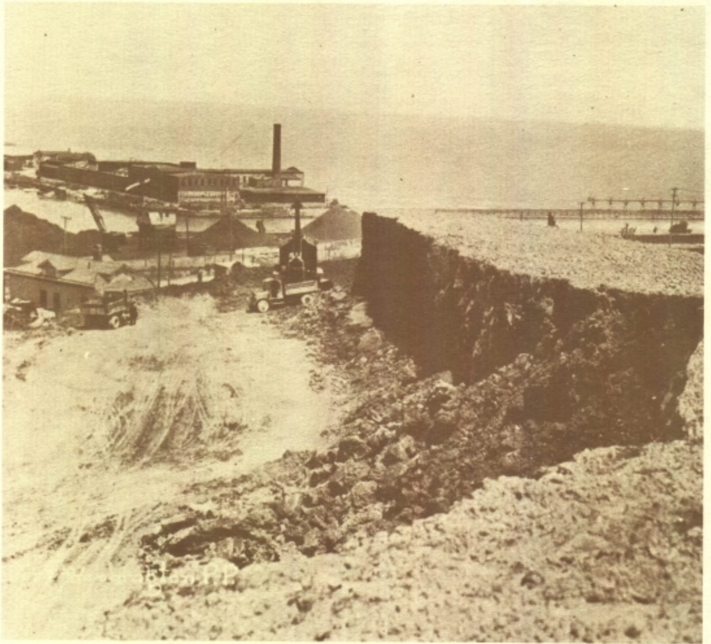
Earth-moving equipment scooped 275,000 cubic yards of dirt out of a bluff on the Lake Michigan shoreline to make room for the plant. The dirt was used to form the fill for the plant's 1,000-foot-long coal dock.
