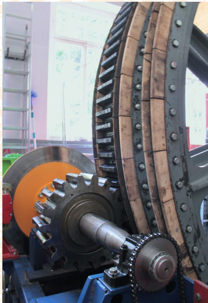
Figure 6: This is the drive shaft. From left to right visible is the service brake disk, the teathed pinion and the chain drive acting for the car position indicator.
