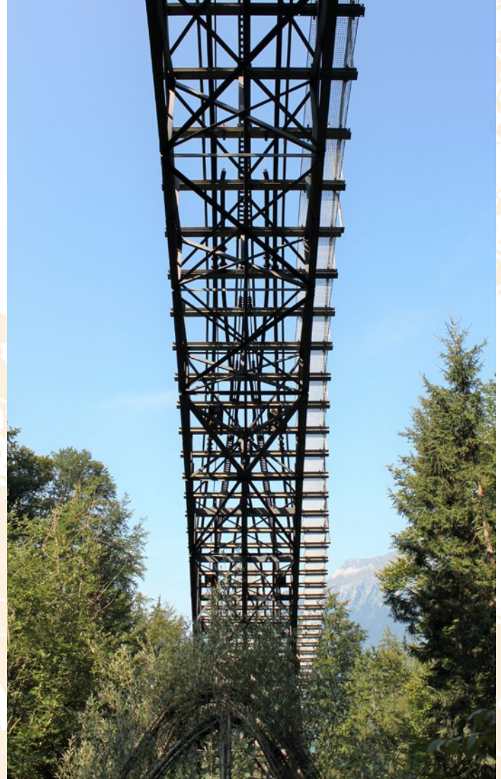
Figure 8: The upper part of the Abt switch seen from below the bridge. The track superstructure is mainly on bridges like this.
